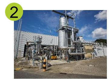
2 Biogas treatment plant
