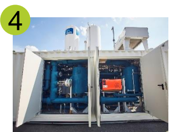
4 Liquefier and e-LNG filling Station
