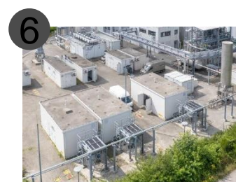
6 Grid injection plant
